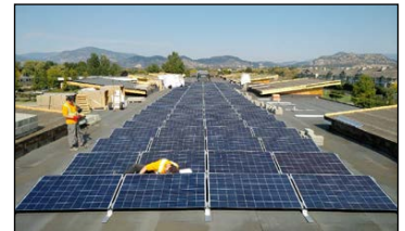
Solar panels at HighStreet's Mission Flats BUILT GREEN® High Density project.
